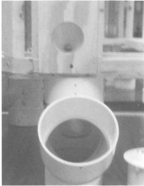
FIG. 10—Close-up of one of the six conduits for removing and servicing ingress jars; the end plug for this unit is shown in the lower right corner.
